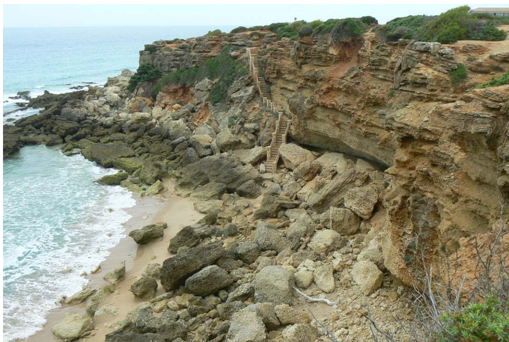
Fig. 6.6. Cliff retreat and rock falls at Cape Roche (Cádiz, Southern Spain).
