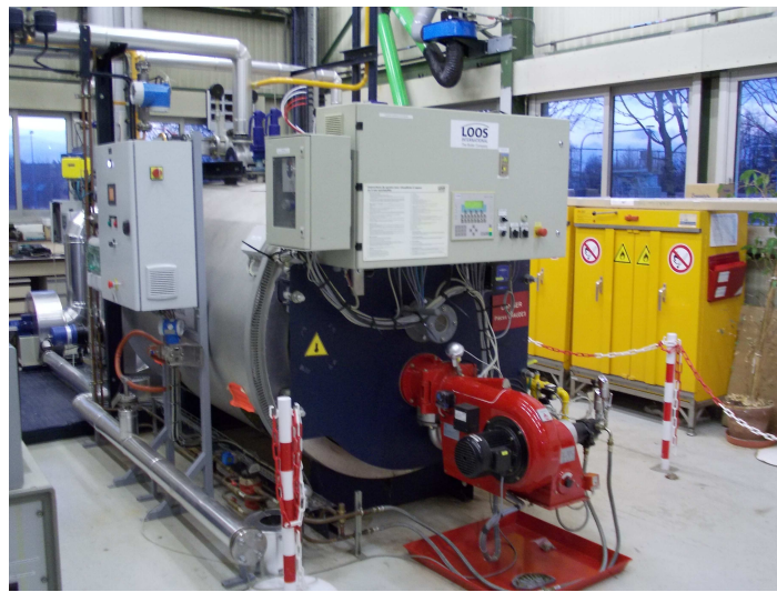
Fig. 2. Boiler side view
