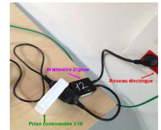
Wattmeter Power Switch
