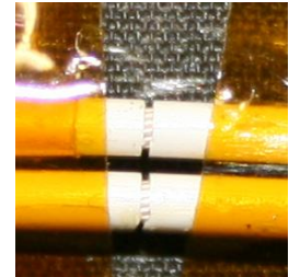
Fig. 2: aged Tefzel® cables. Cracks are due to aging
