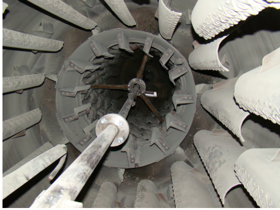
Figure 1 - View of an empty rotary drum used in the Hot-Mix-Asphalt (HMA) plant and equipped with the probes rod.
