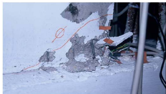
Figure 12. Experimental damage pattern for T5 motion.
