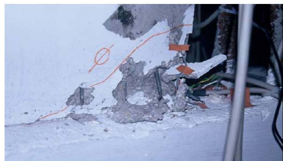
Figure 12. Experimental damage pattern for T5 motion.
