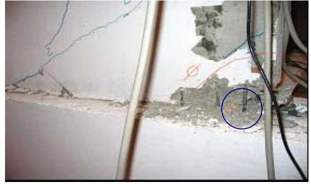
Figure 20: Broken steel at the base of the walls X right (T6)
