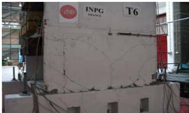
Figure 19. Experimental damage pattern for T6 motion
