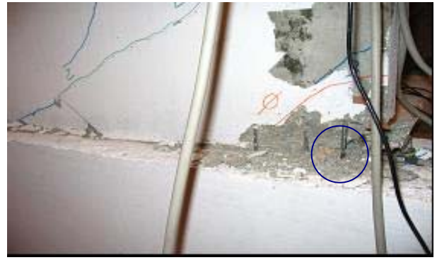
Figure 20: Broken steel at the base of the walls X right (T6)
