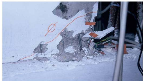
Figure 12. Experimental damage pattern for T5 motion.
