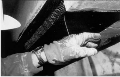
Figure 5.1. Increase of the flexural capacity by FRP bonding on the lower part of a beam.
