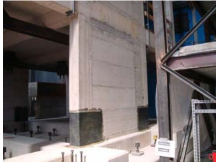
Figure 2.5. Reinforcing of the column with CFRP to safeguard against column lap-splice failure
