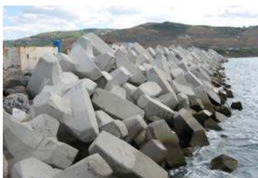
Dike with slope protection constructed from concrete shielding (Protection against ocean swells)
