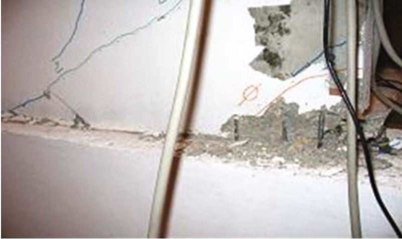
Fig. 18 Broken steel at the base of the wall X right for T6 motion
