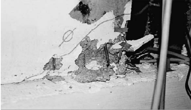
FIGURE 7 State of the XD wall at level T5.
