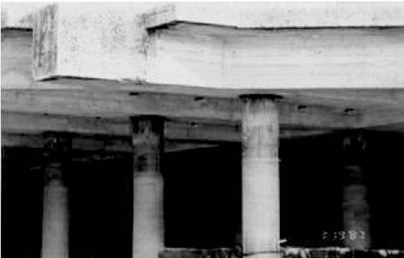
Fig. 6. Steel piles with corrosion.
