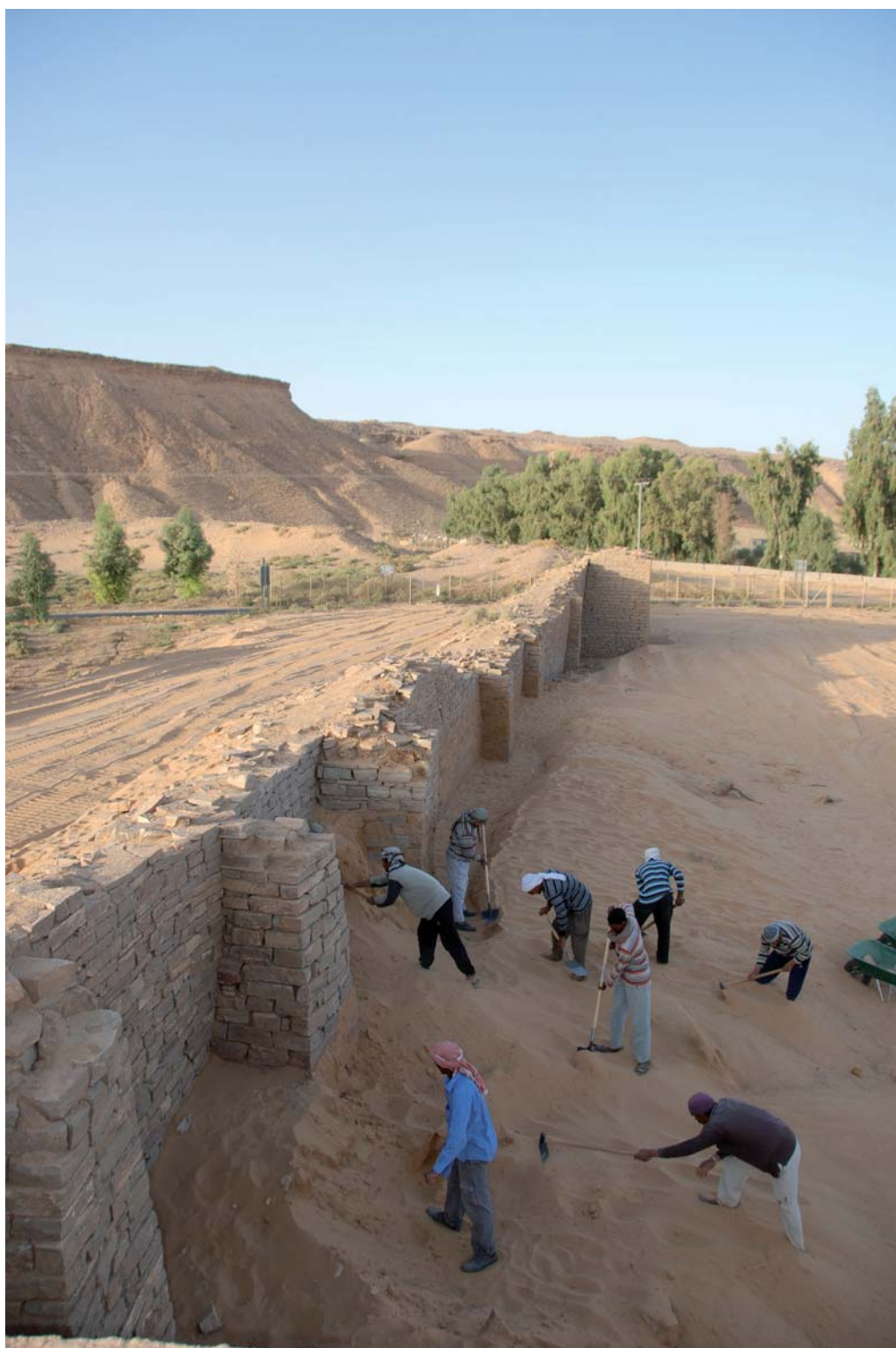
Fig. 80. Cleaning of the western face of the enclosure wall (unit 3) by workers, looking south
