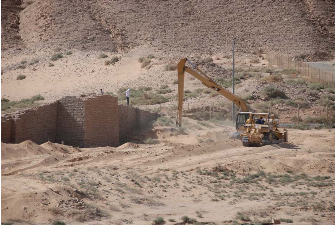
Fig. 79. Clearing of the western area of sector C using mechanical instruments, looking south
