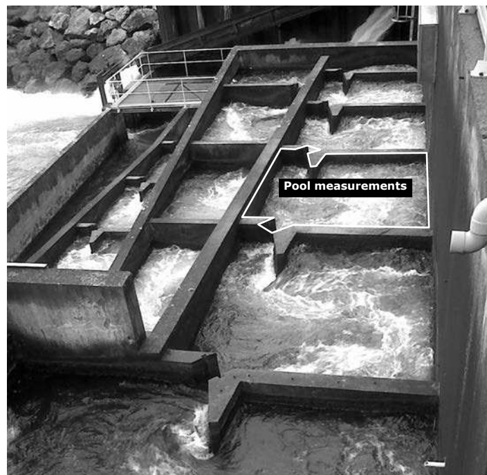
Figure 1. Vertical slot fishway of the hydroelectric power station of Pardies on Gave de Pau River.
