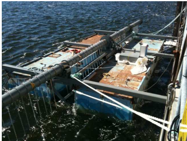
Fig. 11. Chain curtain used for creating turbulence in the intake bay.
