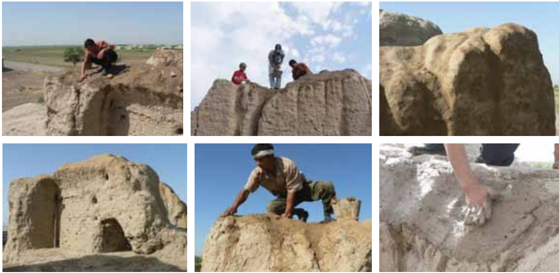
Fig. 2 - Applying sacrificial renders at the top of ruined walls to reduce the speed of erosion
