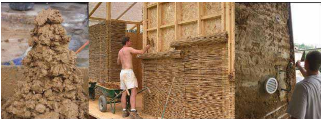
Fig. 6 - Changing earth size distribution by adding sand or gravel and its constructive innovation: Jean-Marie Le Tiec prototypes (© CRAterre-ENSAG)
