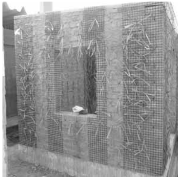
Fig. 6 - Model M075-T11: reinforcement arrangement and model during construction (PUCP shake table tests 2008)
