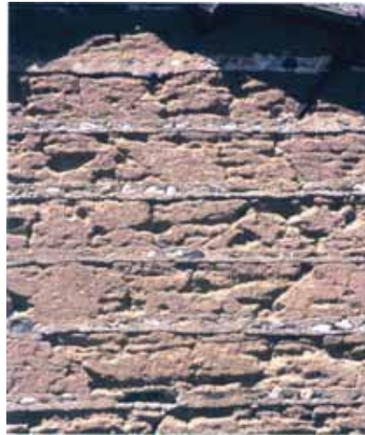
Fig. 9 - Horizontal clamping in a pisé wall from an old farm (18th century) in South-West France (Klein, 1999)
