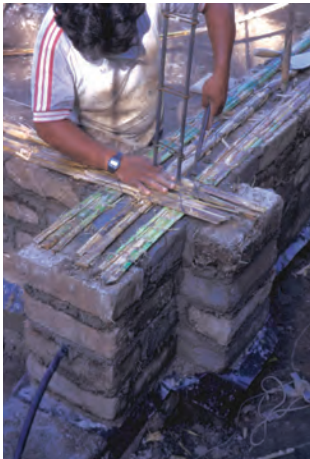
El Salvador horizontal reinforcement paraseismic system
