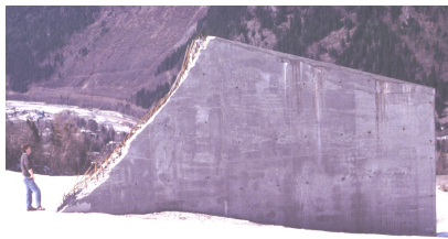
Figure 2: Taconnaz wall partially destroyed in 1999 (photo courtesy of F. Rapin, Irstea)
