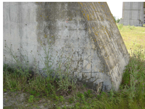
Figure 15: Cracking is more important in the bottom of the base because of the capillary suction (Cheviré bridge)
