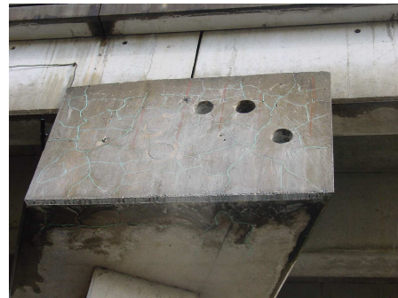
Figure 13: Map cracking at the end of the cap beam exposed to rain
