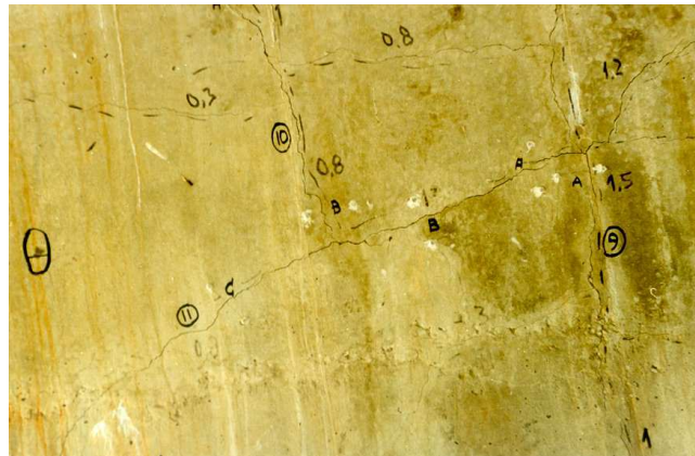
Figure 9: Network of cracks on the cap beam of the North pier
