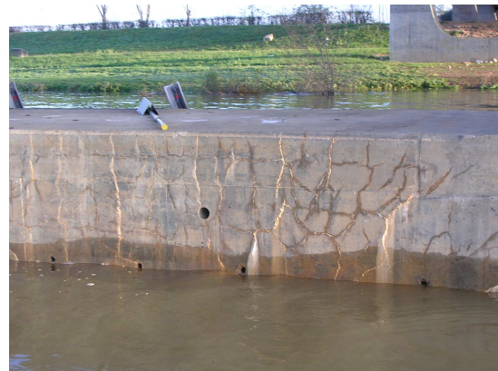
Figure 7: Cracking of the aerial part of the pylon base
