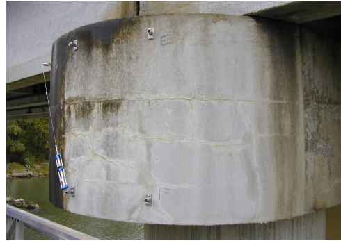
Figure 3: View of the end of the cap beam in 2005, after the treatment applied in 1995
