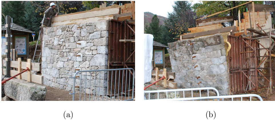
Figure 8: Full-scale field trials of dry-stone walls: preparation before experimentation (a) and overturning of the wall (b).
