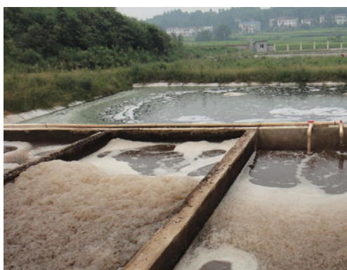
Fig. 5 Wastewater treatment of scaled livestock breeding
