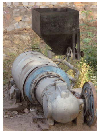
Figure 1. Rice husk-based combined heat and power (CHP) electric generator.
