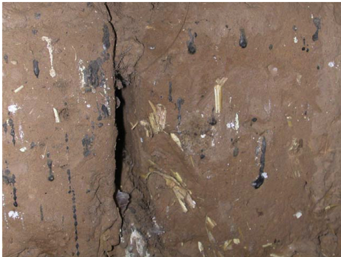
Figure 2. Crack offering refuge to triatomine bugs and fecal streaks in a mud wall. (A color version of this figure is available at www.vetres.org .)
