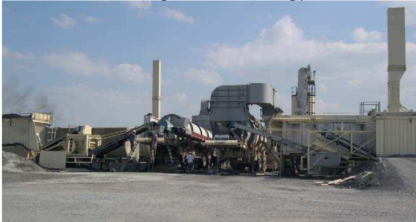
Picture 1 : Benninghoven continue mixing plant 450t/h
