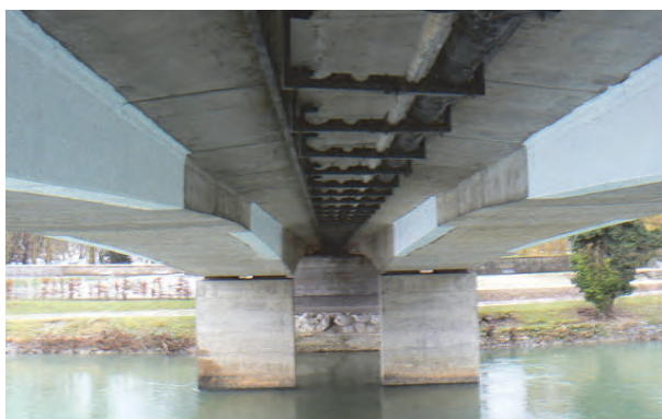
Fig. 17. View of the bridge under consideration; FRP repaired zones correspond to the white parts on the girders.
