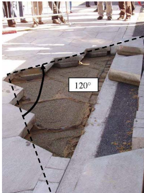
Figure 12: Removal of the connected RUP slab - All slabs within a 120° dihedral must be removed in order to reach any inner point of the pad.
