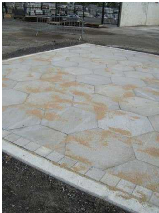
Figure 10: The Nantes RUP after completion (Note the pavers line along the pad edges.)
