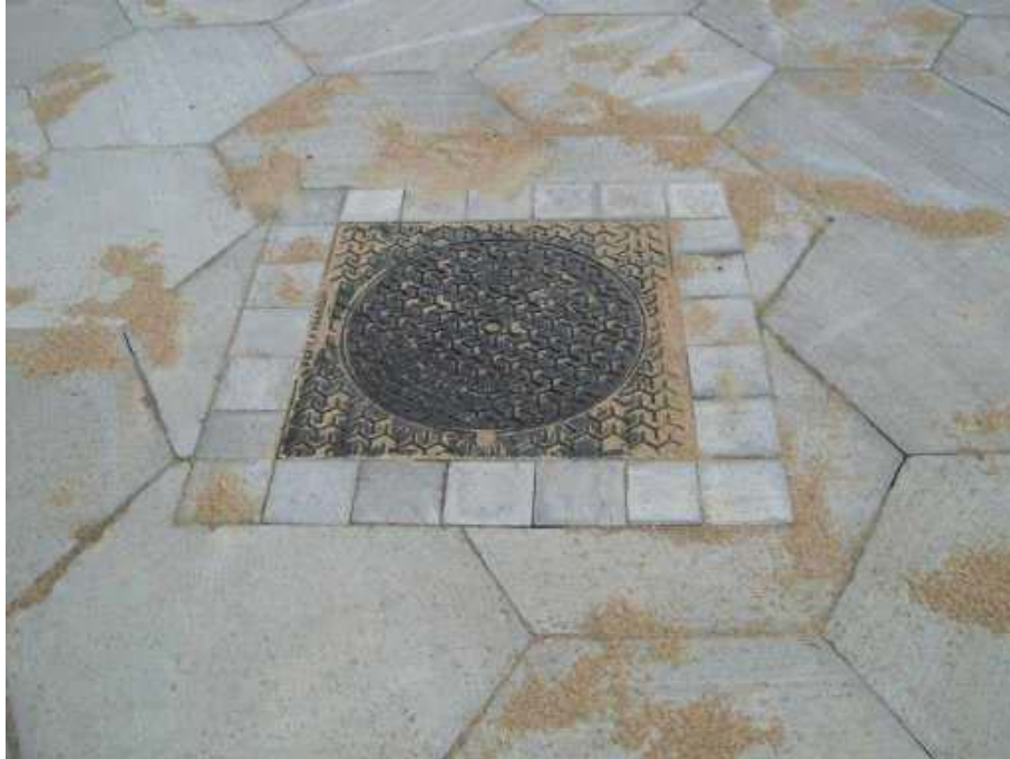
Figure 11: Fixed underground service outlet, surrounded by removable pavers and slabs
