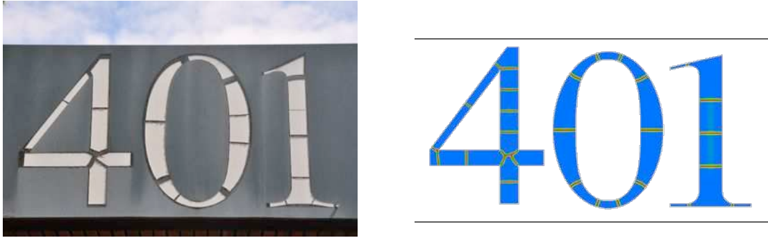
Figure 15: Cracked lettering at École Polytechnique, Palaiseau, France and numerical simulation for t = 1.75 .
