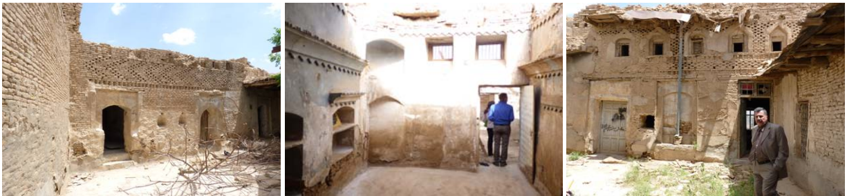
Standing structures requiring conservation work
