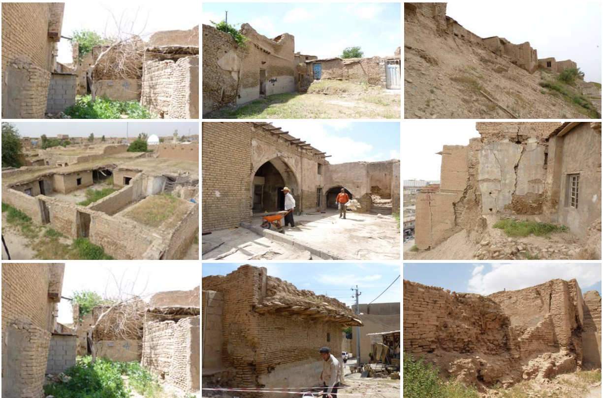
Partially collapsed structures
