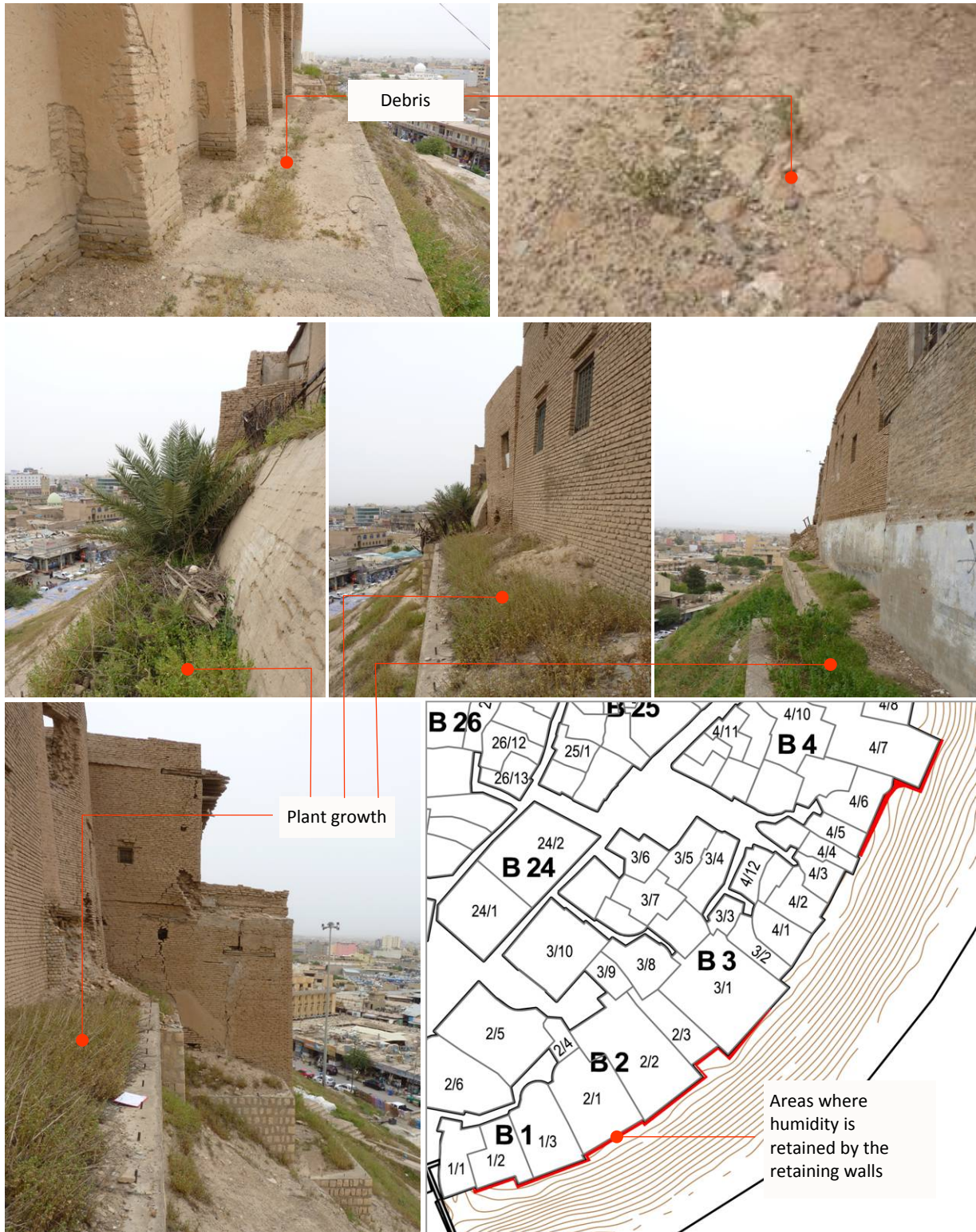
Photographs of the base of the perimeter wall, where retaining walls have been built.
