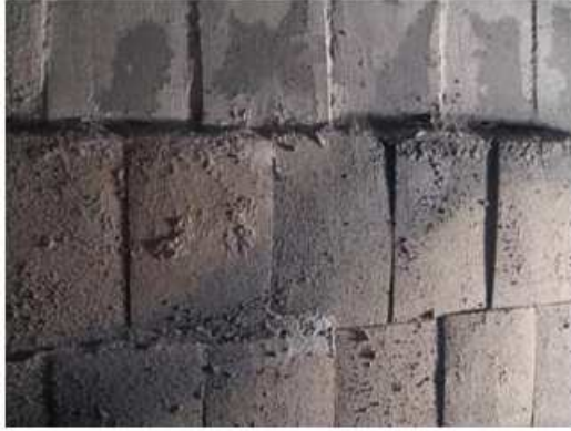
FIGURE 1. New (top) and old (bottom) SiC based refractory tiles in a WTE facility (tile height: 245mm)
