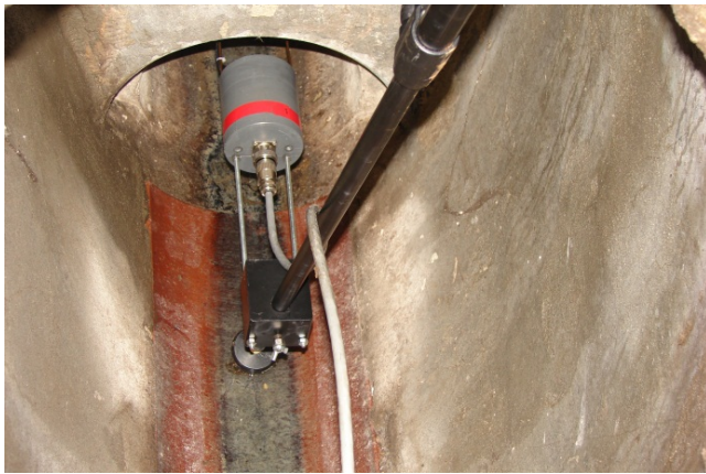
Figure 7: The method for sensor deployment in a live (300mm) sewer in the field.
