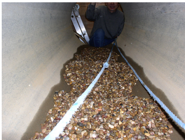
Figure 6: The method for sensor deployment in a live (300mm) sewer in the field.
