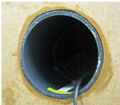
Figure 2: Microflow USP probe, fixed to a frame and inserted into the open end of the pipe
