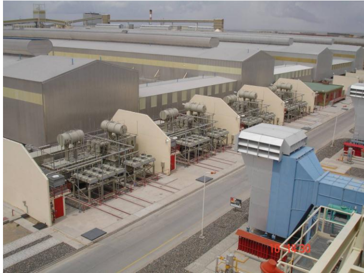
Fig. 1. Example of an AREVA T&D aluminium electrolysis substation: ALUAR (Argentina)
