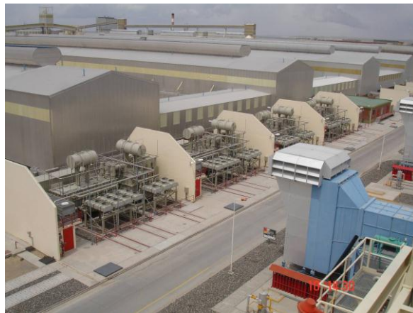
Figure 2. Example of AREVA T&D conversion substation (ALUAR smelter, Argentina)
