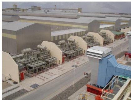
Figure 3. Example of an Alstom Grid aluminium electrolysis substation (Aluar smelter, Argentina)
