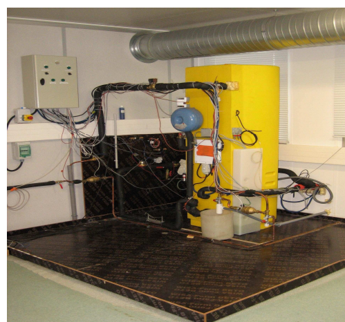
Figure 3 : Storage tank installed in the test space
