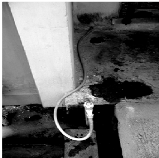
Drinking water connection to a household, Avvai Nagar
