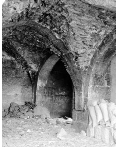
(pic. 15) Han al-Bagrur , Jazirah (south-east Turkey), 1219-20, Ayyubid, court caravanserai. Groin vaults of halls. (2008)
