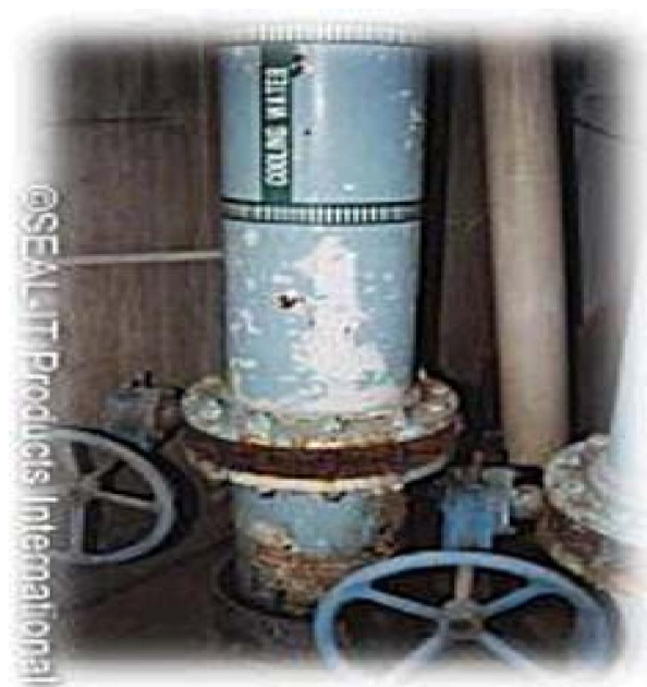
Fig. 3. Crevice Corrosion in a Flange
