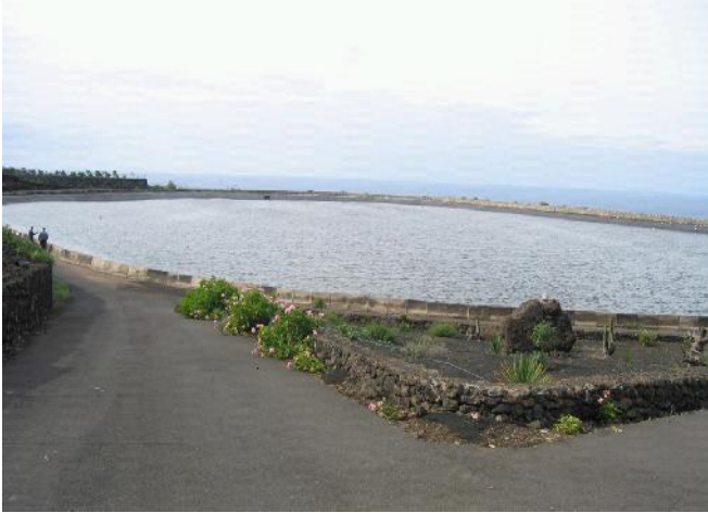
Figure 3. "El Golfo" reservoir which is waterproofed with an EPDM polymeric geosynthetic barrier.
