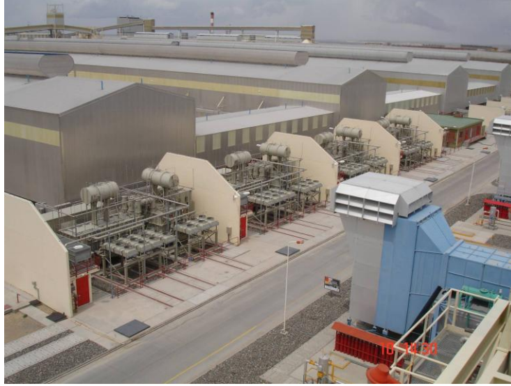
Figure 4. Example of an Alstom Grid AC/DC conversion substation (Aluar, Argentina)
