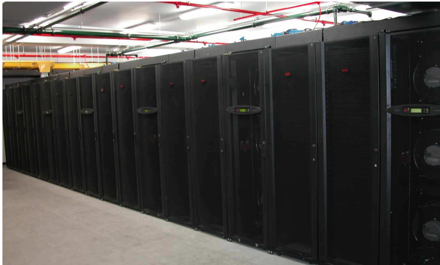
Figure 3.1: GRNET datacenter hosting StratusLab’s infrastructure
