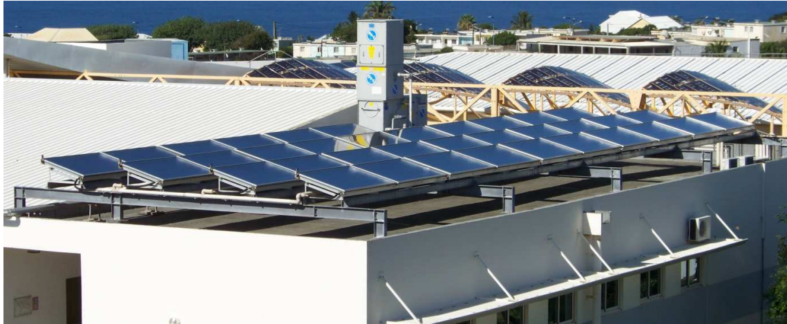
Fig. 4 : Solar collector field of the solar cooling process
