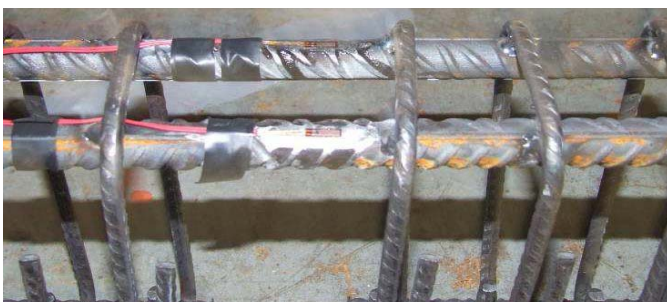
Figure 3*. Strain gauges attached to the steel bars at mid span. *view before the pouring of concrete.
