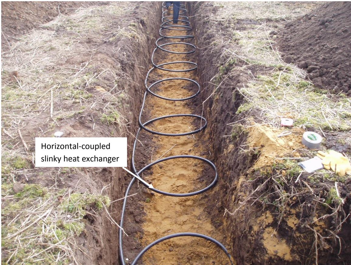
Figure 1 Image of the horizontal-coupled ground source heat exchanger at Talbot Cottage, Drayton St Leonard site, Oxfordshire, UK
