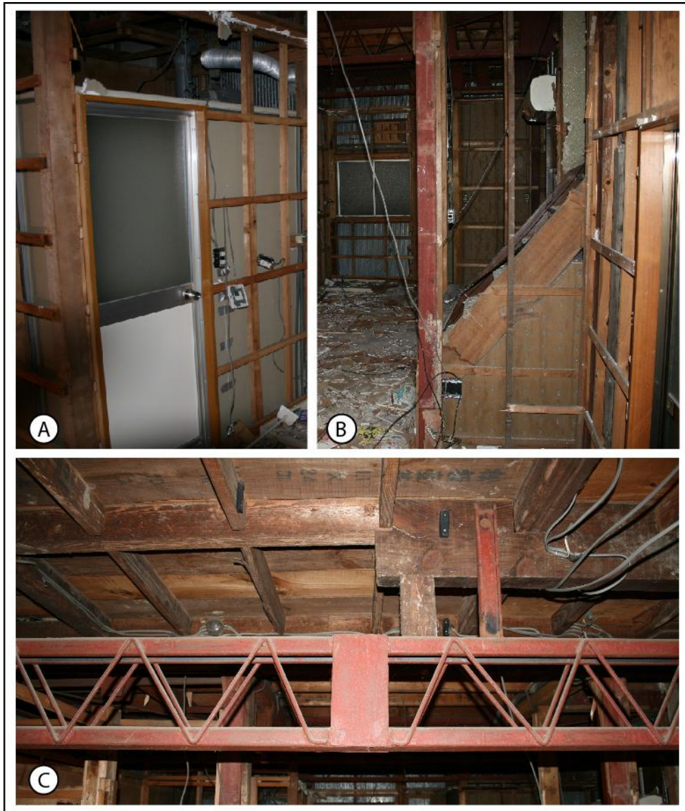
Fig. 8 Typical timber-frame structure house, which has been reinforced by a metallic structure during the Showa period (1926-1989). We can also appreciate the external wall panels made of painted steel. (Photos: C. Gomez, 2006)
