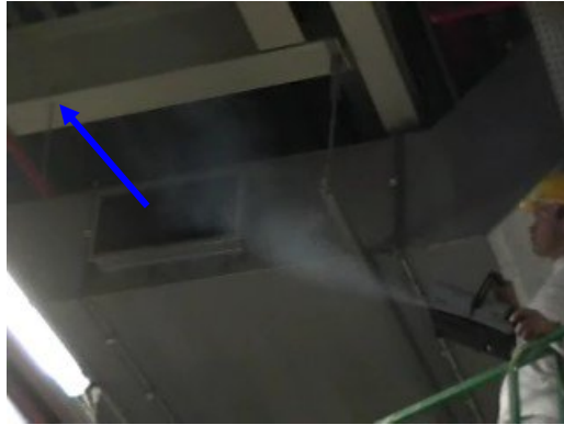
Figure 6 - Smoke injection at duct level.
